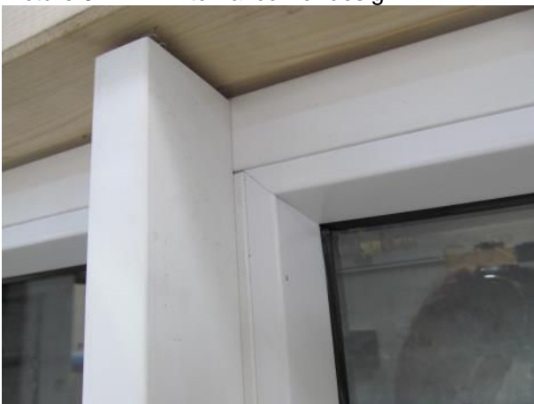
Picture 5 Central meeting joint, at top
