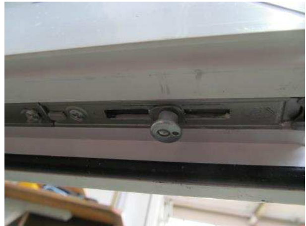
Picture 14 Locking situation, casement 2
