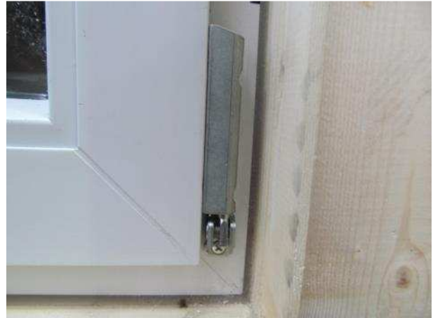
Picture 8 Corner pivot, seen from inside
