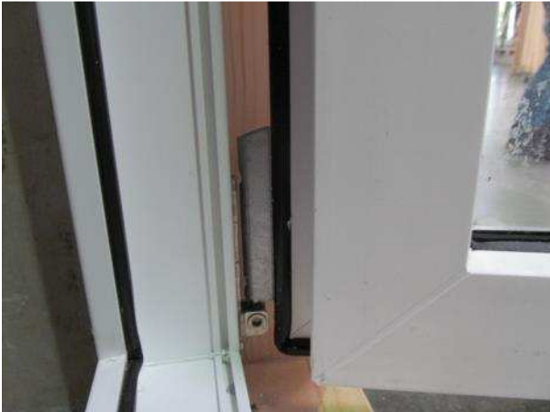
Picture 7 Corner pivot, seen from rebate, frame
