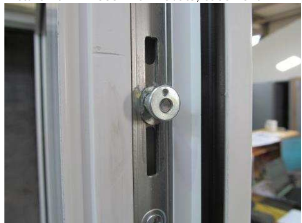
Picture 12 Locking situation, casement 1
